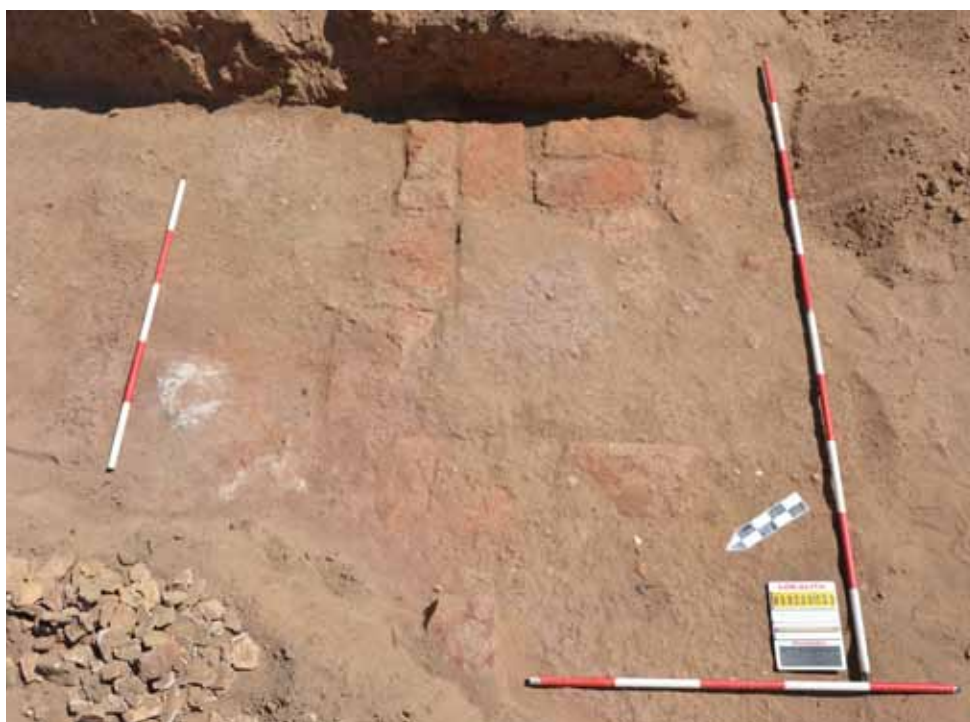
Pl. 4 Foundations of the western Bes pillar of the southern pair of pillars in the Typhonium (Photo: Alexander Gatzsche).
