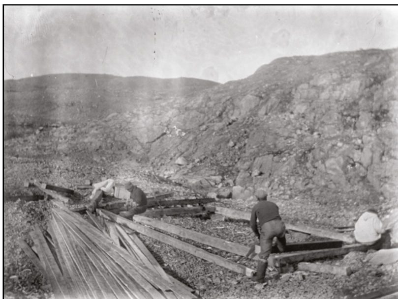
Pl. 14. Construction of house foundations. Canada, Labrador, b/w negative glass 90 × 120 mm, Inv. No. Am I 6607. (Photo: Jiří Jaeger, 1914–1919).
