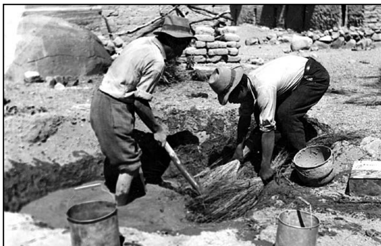
Pl. 36a-c. Roof thatch covering procedure, Enquelga, Chile. Václav Šolc, 1968. Roll film negative 60 × 60 mm, Inv. No. Am I 2007.
